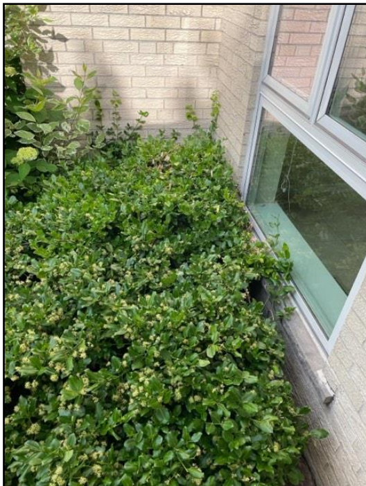
Shrubs- too close to building...
